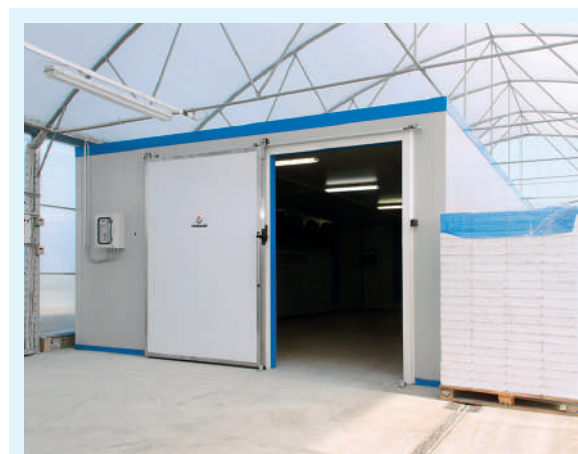
Germination chamber installed in a warehouse.
