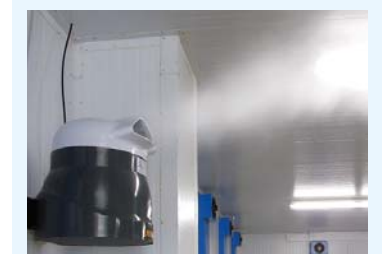
Humidifier in operation inside a germination room.
